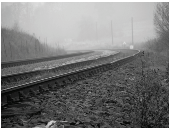
Fig. 1. View of the track number 1NA line PKP PLK No.286 Main Station Kłodzko – Wałbrzych. Source: M. Winiarski [3].
