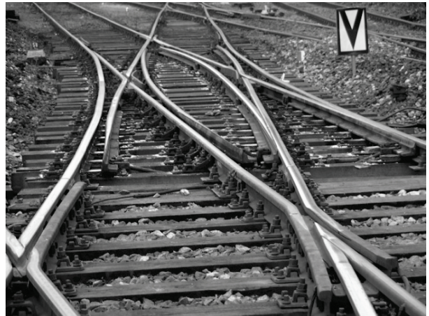
Fig. 4. RKPd S60 (E1) turnout after replacing the bearers, without exchanging crushed ballast (Example of the main non-complex repair).
