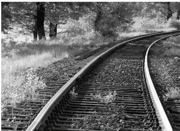
Fig. 3. A fragment of railway track No. 279, prepared for the exchange of rails.
