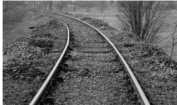
Fig. 7. A state during the repair of the track on the PKP line Luban – Lesna, after a train derailed.
