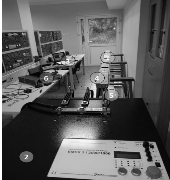
Fig. 7. Lab stand: 1 – bus bar system, 2 – three-phase current supply, 3 – PC with measurement software, 4 – magnetic field probe (inside the shield), 5 – Rogowski coils, 6 – additional measuring equipment (voltmeter, phase meter)
