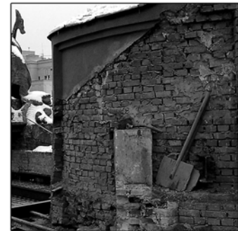
Coursed brick masonry of the early 20th century (The House with Chimaeras)
