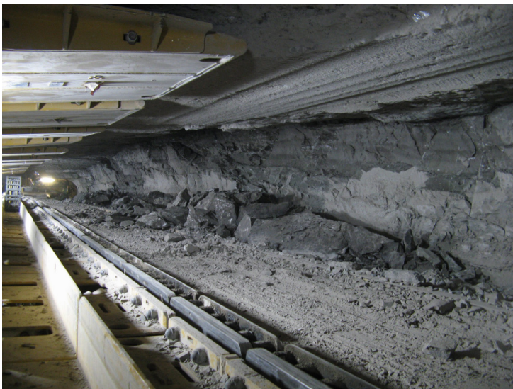
Figure 17: Examples of failures that occurred in the 5A/1 longwall: a, b) roof falls, c) wall spalling.
