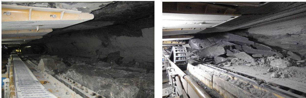
Figure 1: Failures in the 5A/1 longwall a) roof falls, b) wall spalling.
