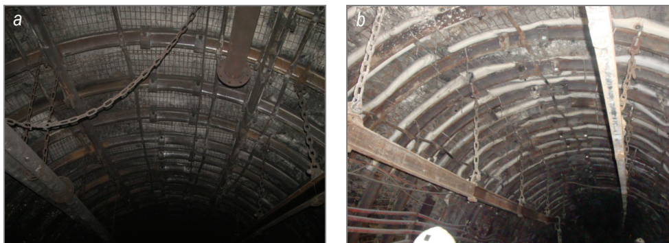
Fig. 2. Support of the bottom gate K-2: (a) support with mechanical lining, (b) support with traditional lining
