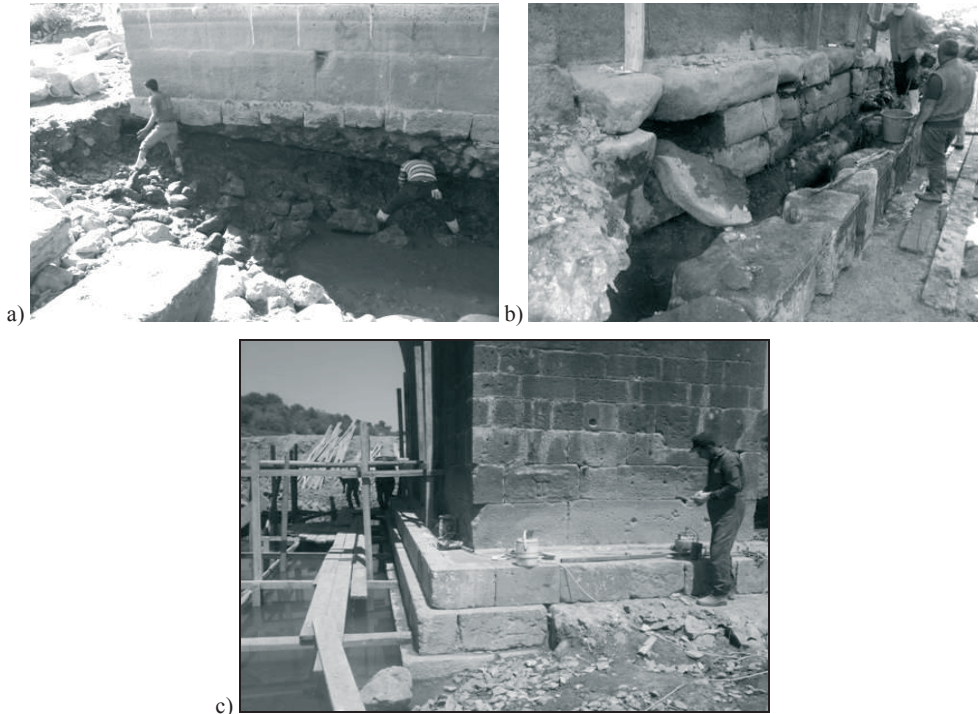
Fig. 5. Conservation works a) discharges on the grounds b-c) splits, cracks and breakages
