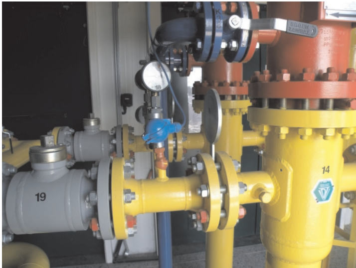
Fig. 2. Transducer of natural gas temperature after the heat exchanger Phot.: Authors
