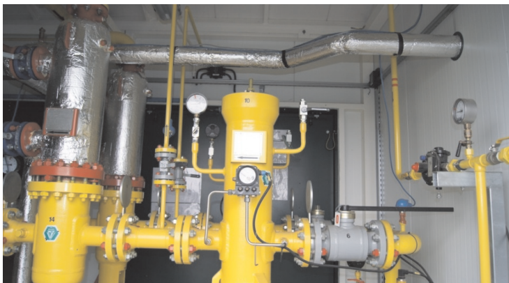
Fig. 4. View of thermally insulated gas heaters and pipelines Phot.: Authors
