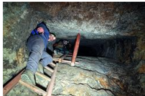
Fig. 8 Employee - excavation of vertical works Source: Author's results by internal company material.
