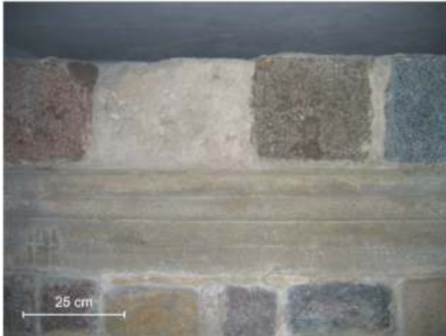
Fig. 6. Poznań, Ostrów Tumski; the basement of Poznań cathedral; a piece of pillar II of the Romanesque church; starting from the upper left corner: granite, calcareous sinter, granite, granite, in a large slab of sandstone from Brzeźno
