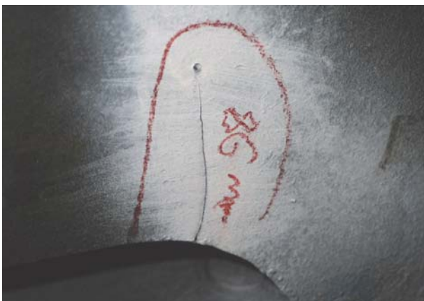
Fig. 4. Crack type P 7 86 mm through the transverse rib detected by the magnetic powder inspection method
