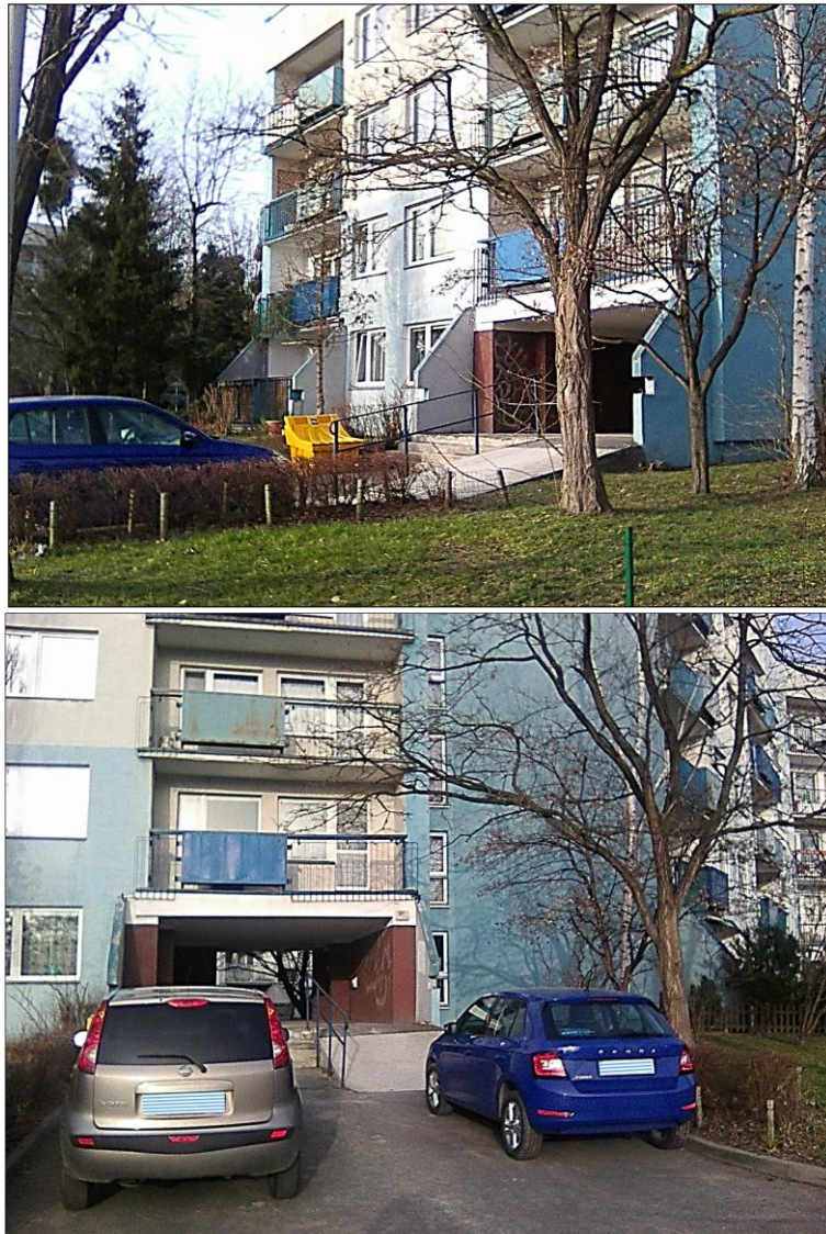
Fig. 3. Main entrance, in low-rise residential buildings, located more than 0.6 m above the street level with a driveway for disabled people, stairs and a ramp without external railings and in poor condition with uneven damaged surface, blocked with parked cars and of a utility container standing in front of the stairs - Kozanow estate in Wrocław (author's photo, 2021)
