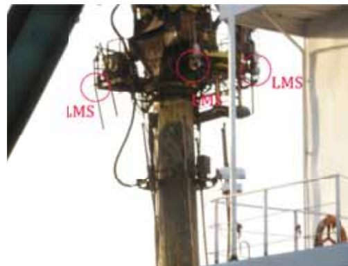
Fig.2 LMSs installed on the ship loader in Tianjin Port
