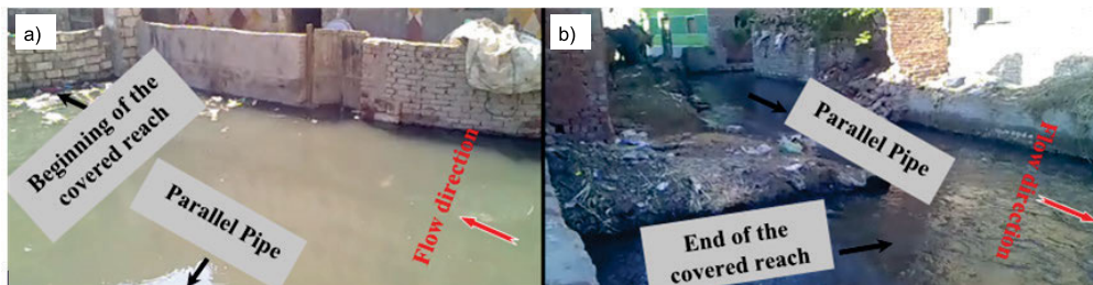
Fig. 4. The Bahr Sanhoor Canal at the covered reach: a) upstream view; b) downstream view, source: own elaboration (camera's photo)
