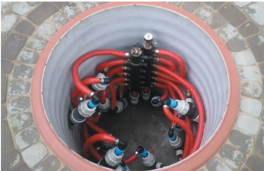
Fig. 10. A ready chamber with a complete installation [2]
