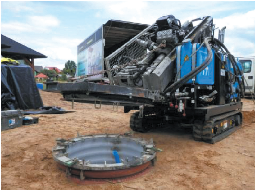
Fig. 2. Preparation prior to the integration of the drill rig carrier and the drilling chamber [2]
