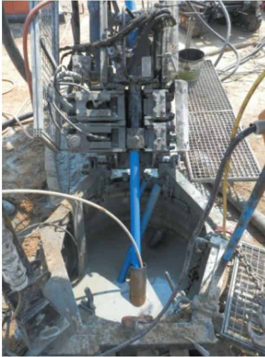
Fig. 9. Inserting the exchanger with an injection pipe [2]
