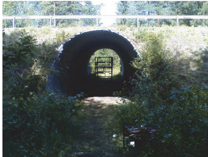
Figure 1. Flexible culvert in northern Sweden built 1966. Measurements under live load were performed in 2012 recording crown deflections and steel strains.
