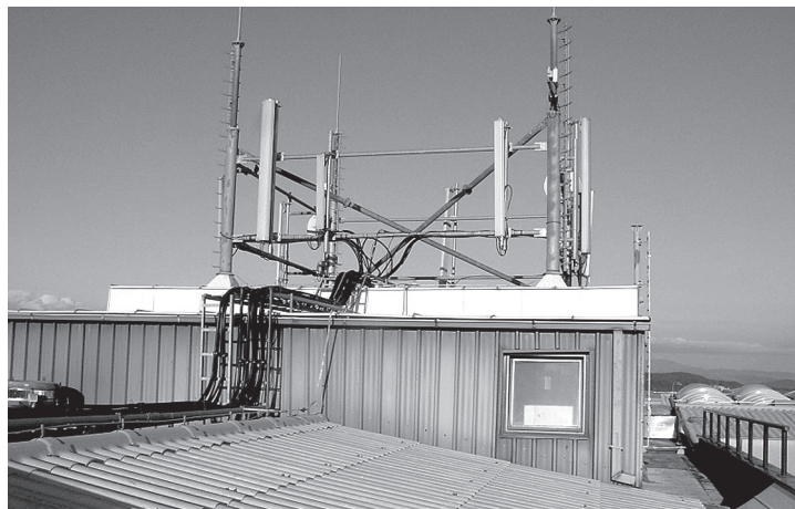
Figure 1. Roof top location of the investigated base station.
