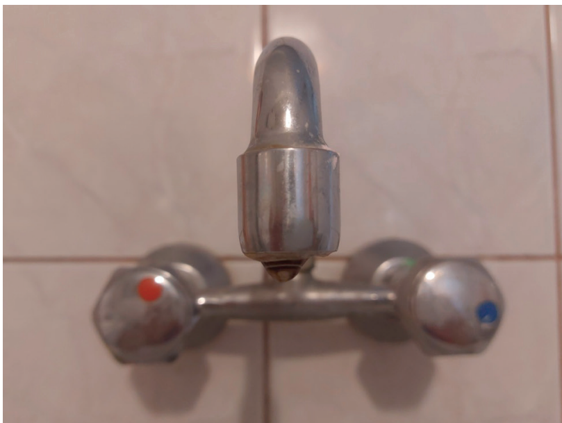
Fig. 7. Water leakage from the sink faucet due to damaged rubber seal
