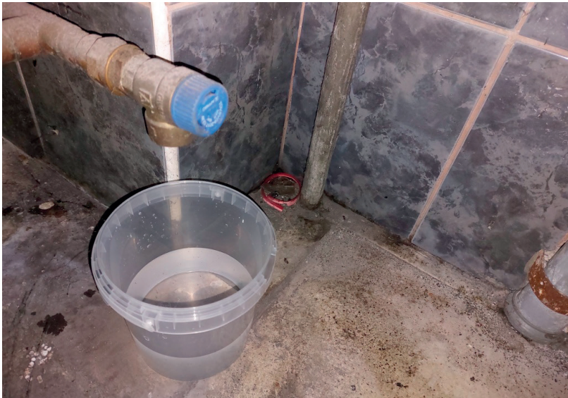
Fig. 3. Water leakage through the hot water tank safety valve (system without expansion vessel)
