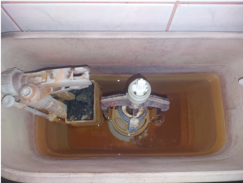
Fig. 4. Water tank with the mechanism covered with limescale
