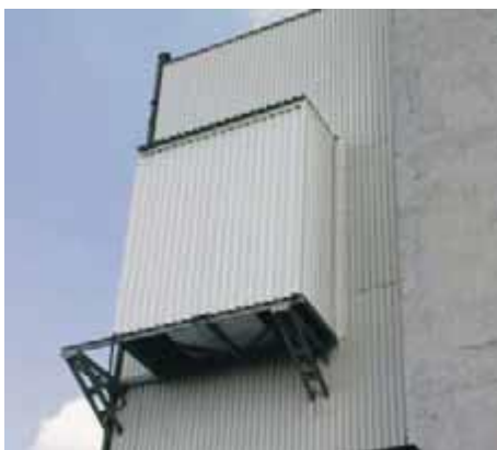
Fig. 18. Silencer of the air draw and ejector installed at the Jankowice Mine [17]
