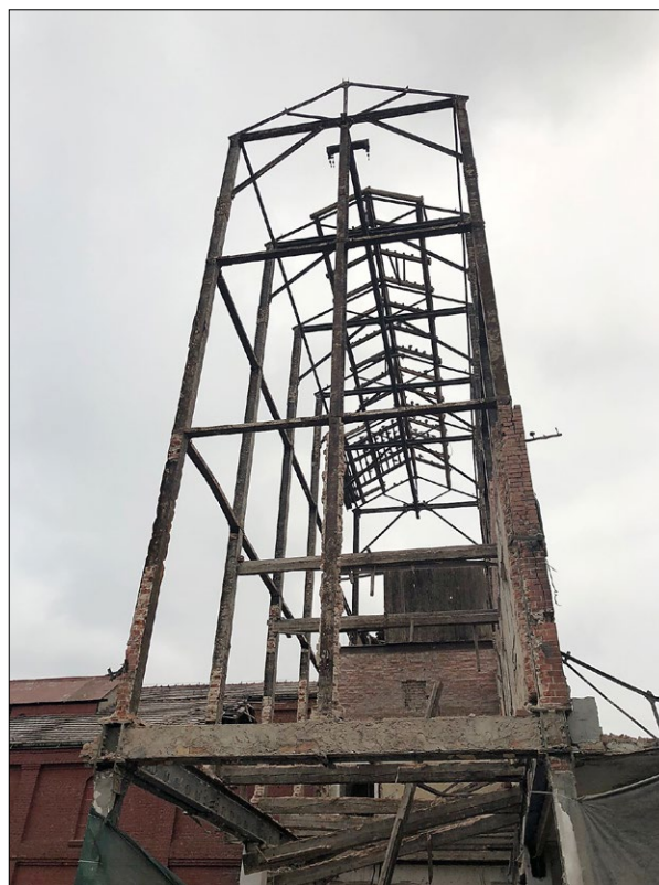
Fig. 5. The high section during the demolition of the deformed and cracked walls with visible corroded steel structure; photo by P. Paradziński.
