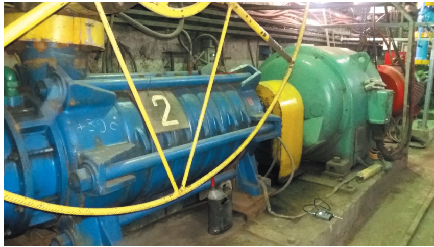
Fig. 2. Pomp unit no. 2
