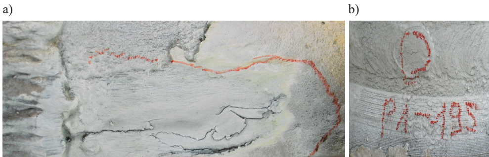
Fig. 2. Cracks detected by magnetic-powder method in area of welded joints of pipelines: a) cracking of native material in direction of pipe axis starting from peripheral weld [7]; b) bursting in perimeter weld [8]
