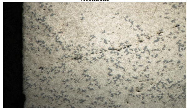
Fig. 6. Total cracking of sample by deflection of 0.2 mm
