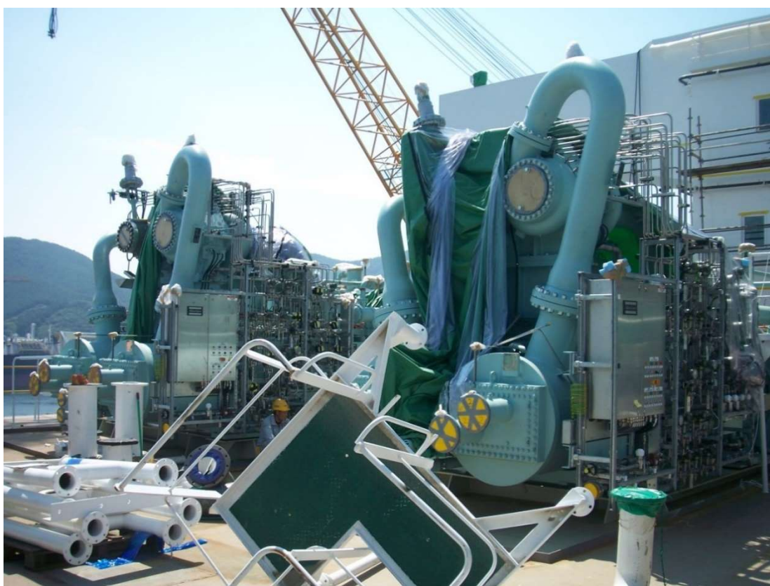
Fig. 3. Atlas Copco nitrogen compander (2 pieces) before installation.
