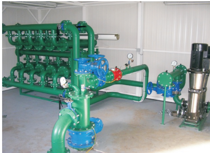
Fig. 6. Injection plant: wellhead, filters, pumps
