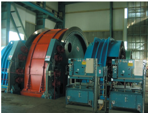
Fig. 1. View of hoisting machine in section (S) of R-II shaft after modernization in 2004 [1]
