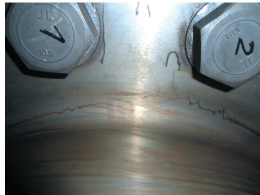
Fig. 3. Cracks on circumference and radial cracks [1]
