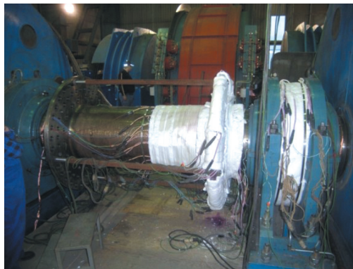
Fig. 6. Area around place of welding was isolated and then heated up with electric heating unit and heating mats. Heating speed was about 25^{\circ}\text{C}/\text{h} [1]
