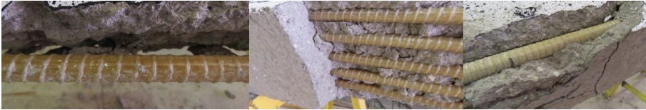
Fig. 3. The outcrop of bottom reinforcement in beams G-512-35-15, G-512-35-35 and G-418-35-15
