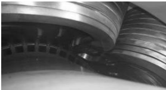
Fig 10. On site implementation (from top): New connector in position, Inductor in place, Final repair effect
