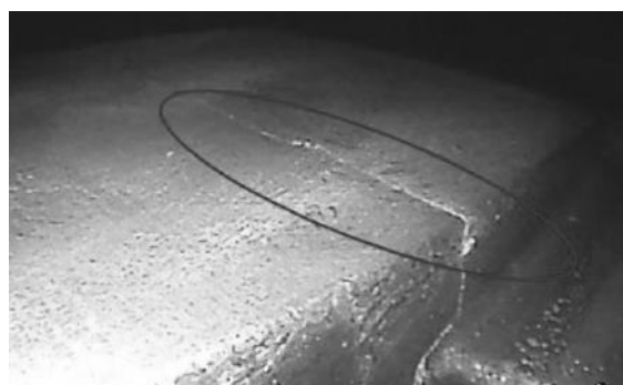
Fig. 2. Exemplary finding in the pole to pole connection during planned inspections
