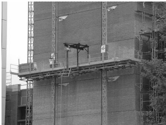
Figure 2. A HEK (USA) climbing platform at about 30 feet (10 m) vertical height. Notes. Brick cut-out for fastening to wall. Brick will be replaced as final operation before removal of platform.
