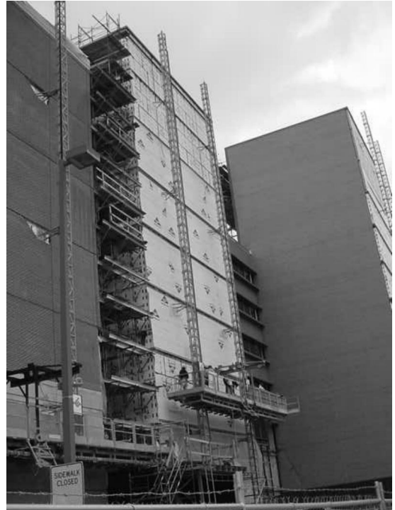
Figure 3. A HEK (USA) climbing platform at about 20 feet (7 m) vertical distance with workers on board.
