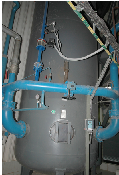
Fig. 4. Compressed air tank (part of a process installation) located in a production building in a power plant
