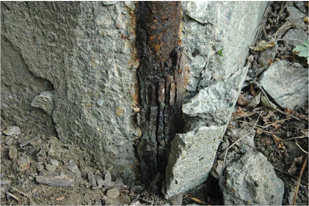
Fig. 4. South pillar of the eastern pier – visible losses of concrete coating and advanced reinforcement corrosion
