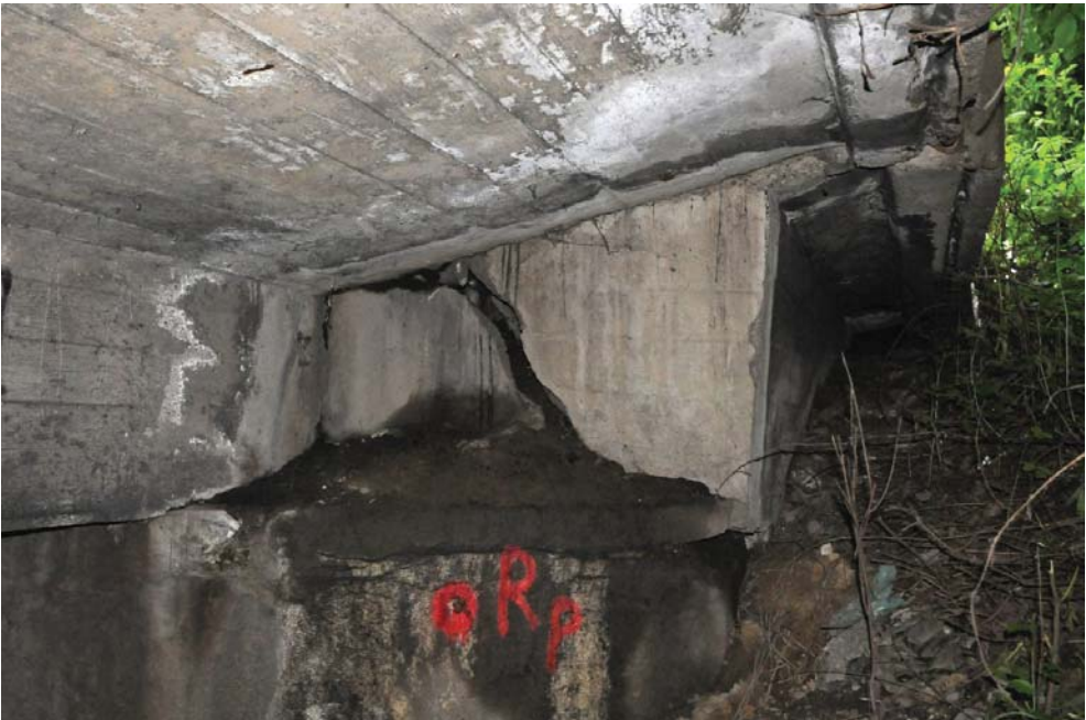
Fig. 5. Western abutment, north side – visible crack of the back wall and dislocation of broken off parts towards the outside
