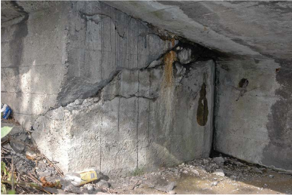
Fig. 6. Western abutment, south side – visible crack of the back wall and chipping of concrete
