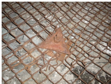
Fig. 5. Corroded parts of a rock bolt support in long-term excavation (photo by K. Skrzypkowski)
