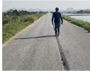
Fig. 3. The location of the levee subsidence on the left bank of the Hoang Long River
