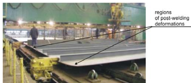
Fig. 1. Welding deformations of a plate section
