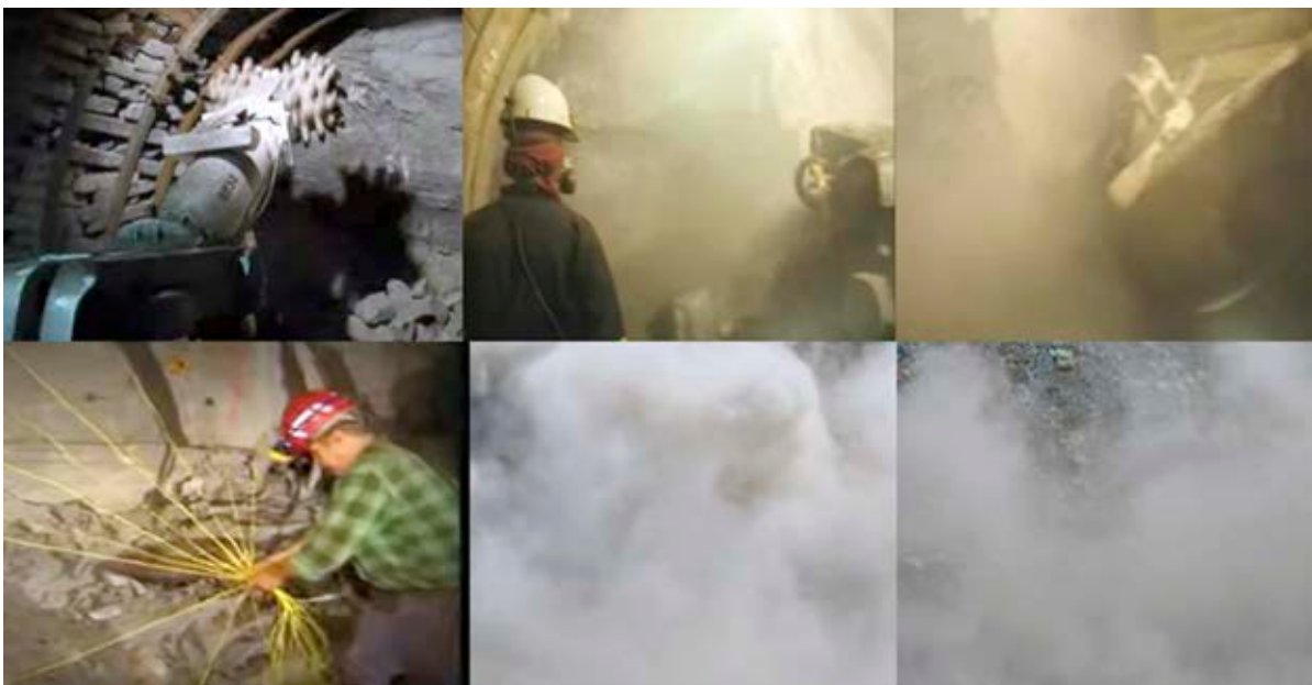
Figure 1. Dustiness during mine face works with the use of the AM-50 roadheader and explosives
