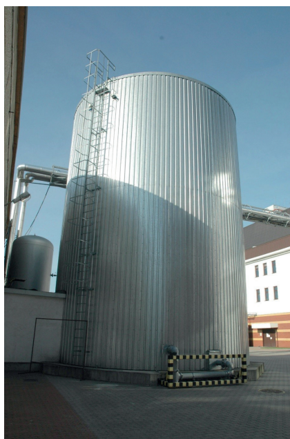
Fig. 4. Fire water storage tank at the industrial plant – the storage tank and the foundation on which it rests are structures
