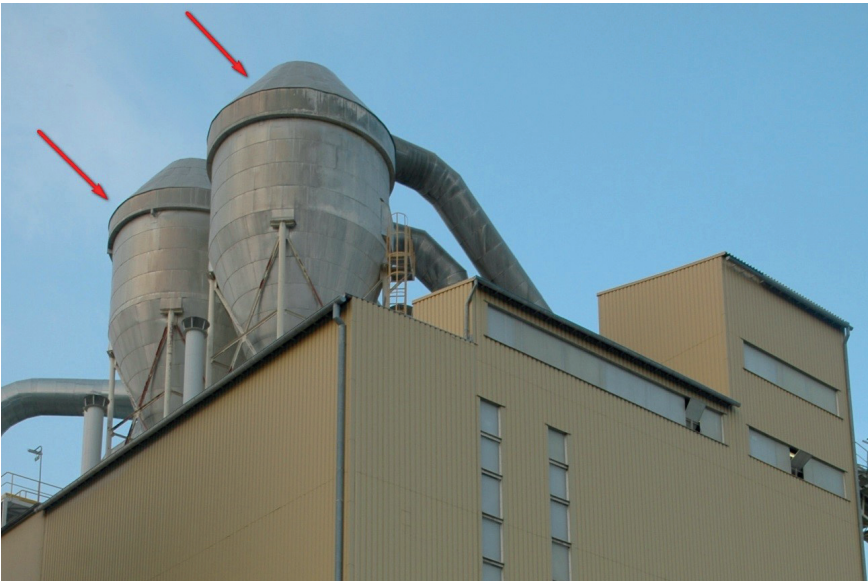
Fig. 7. Dedusting system tanks – elements of the process equipment based on the process facility at the industrial plant
