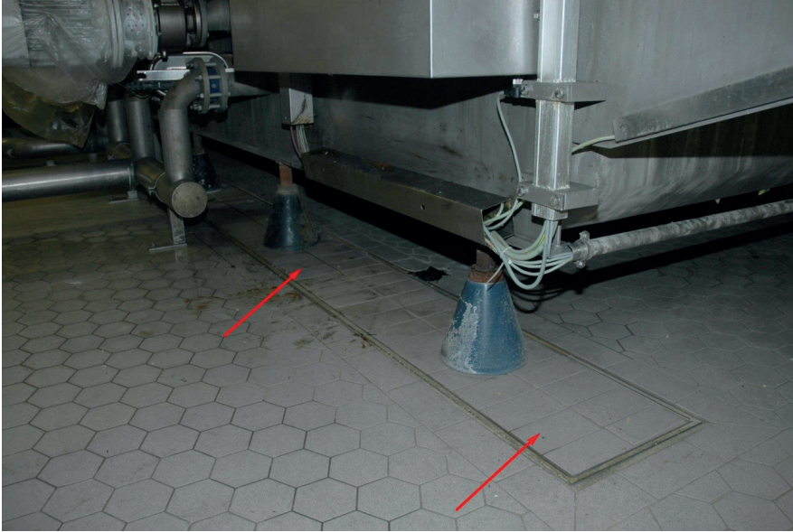
Fig. 12. Fragment of the beam foundation of the device located in the industrial plant production hall – the object is not the structure
