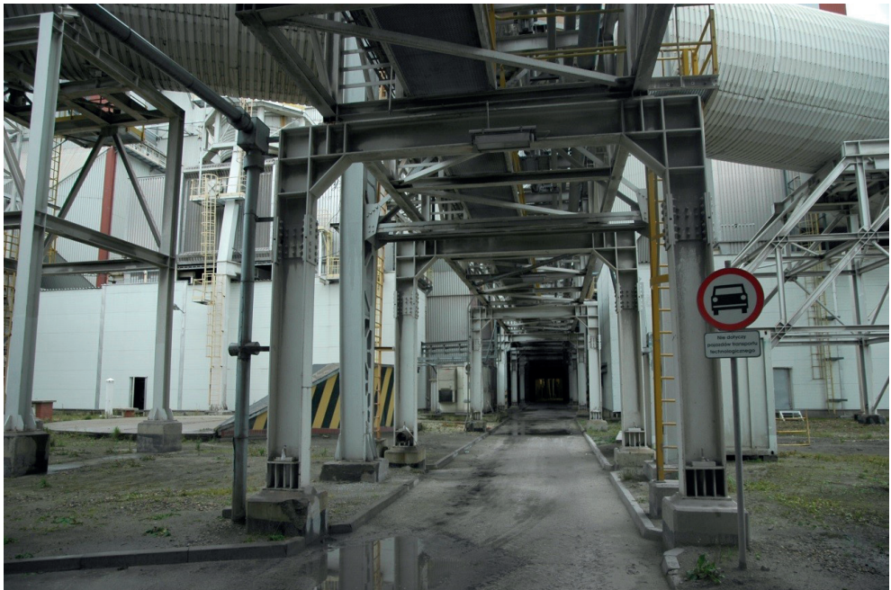
Fig. 8. Fragments of the engineering flyover with a steel frame structure. There are cables and pipelines on the flyover which are elements of the engineering process implemented in the plant – only the flyover is the structure
