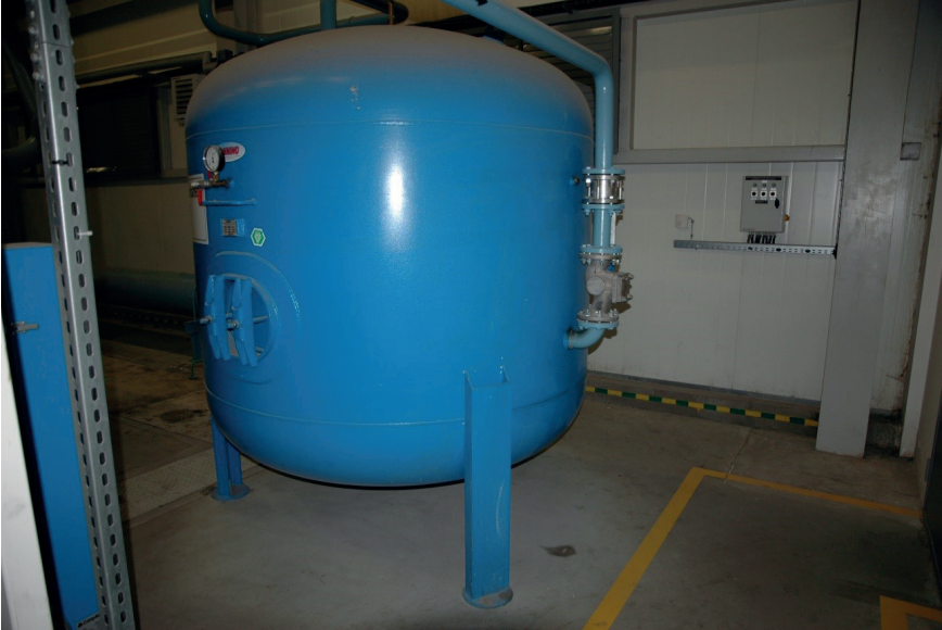
Fig. 6. Compressed air tank – elements of the process equipment resting on the floor in the process facility of the industrial plant
