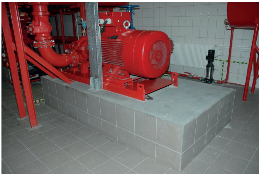
Fig. 11. Block foundation of the pump, located in the warehouse of the industrial plant – the object is not the structure
