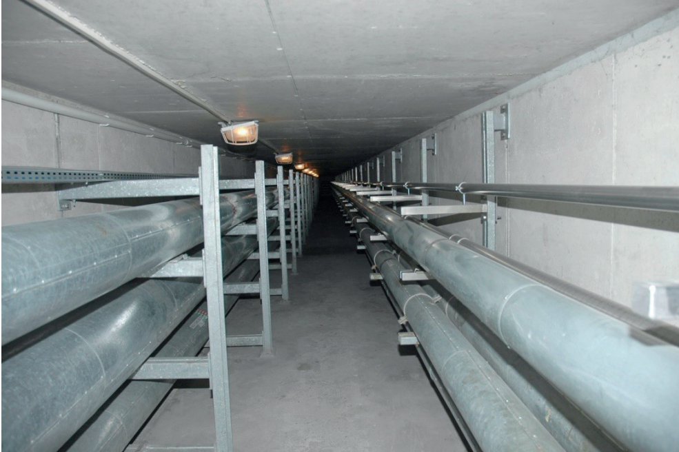
Fig. 9. Engineering duct between production buildings in the plant. The duct contains pipelines which are constituents of the engineering process implemented in the plant – only engineering duct is the structure
