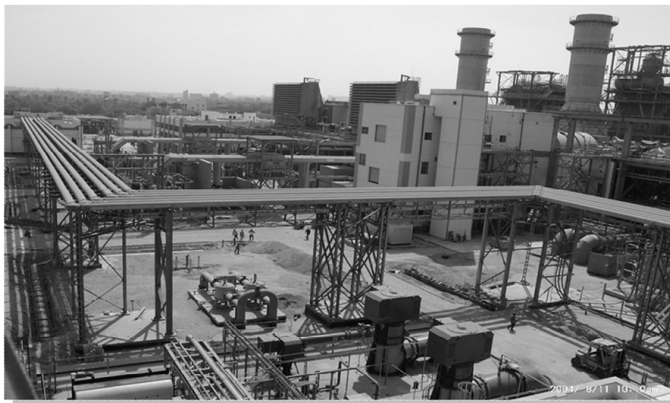
Fig. 1. 245 kV GIL Cairo North [9]
