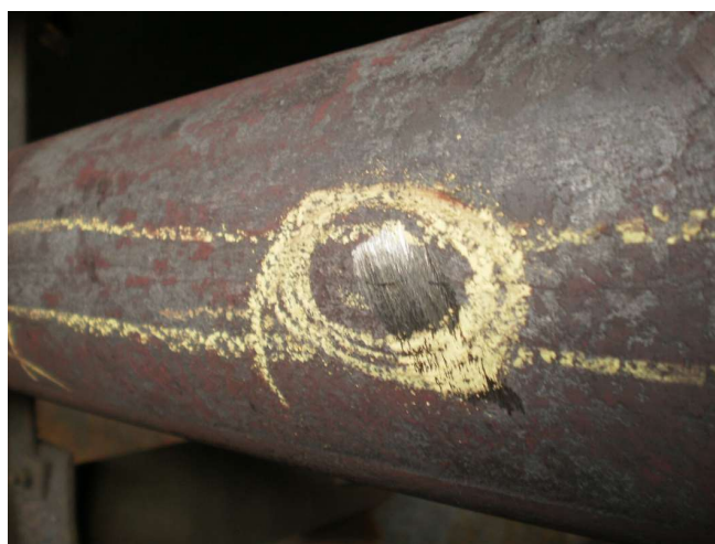
Fig. 4 Crack on the outer surface
