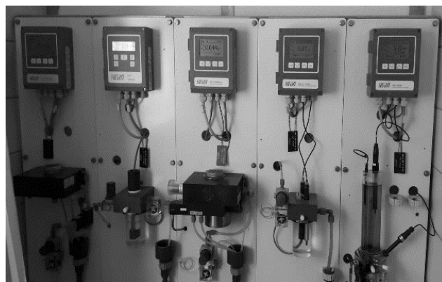
Photo 1. Automatic dosage and monitoring of chlorine concentration in water for disinfection and monitoring the kinetics of water reactions (phot. V. Beluli)
