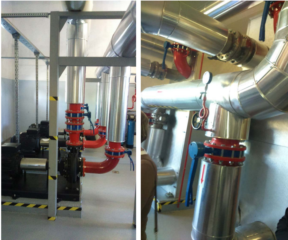
Fig. 1. Poddebice Heat Central; circulation pumps (left) and heat exchangers (right)
