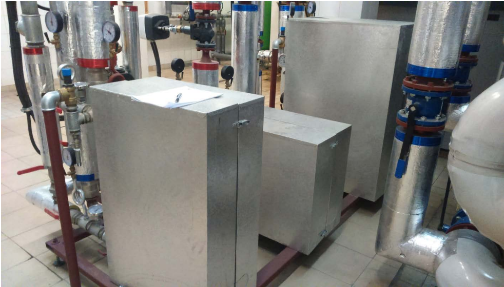
Fig. 2. Heating central at Municipal Health Centre in Poddębice
