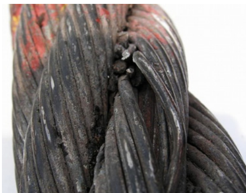
Fig. 1. Example of clearly visible damage to the rope in the form of broken wire
