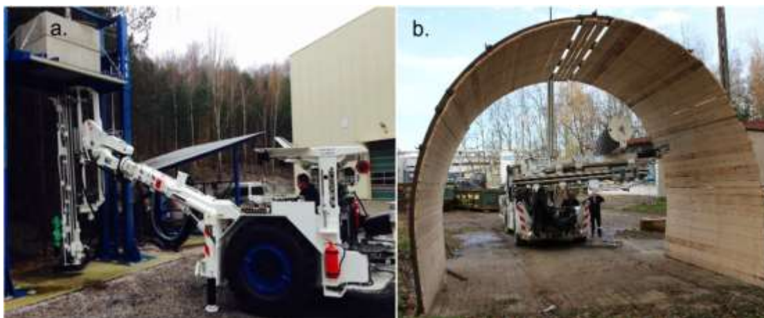
Fig. 11 Verification of the functional properties and parameters of machines at workstations: a. Roof Master 1.8 AWKM anchoring, b. installation of Roof Master 2.3 grid in an artificial tunnel
