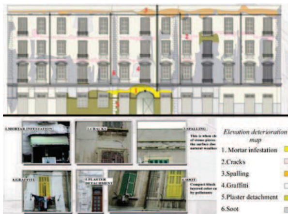
Fig. 15. Different types of deterioration on wekalet El-Lamoun main façade
