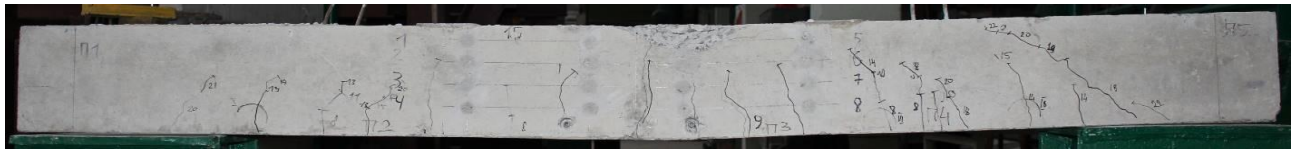
Fig. 6. General view of tested beam BC with common cracks marked
