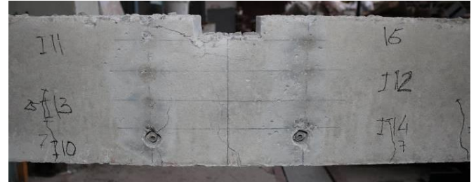
Fig. 10. Display of generated cracks and chips in beams BD.80-0.3
