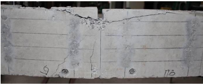
Fig. 8. Display of generated cracks and chips in beams BD.20-0
