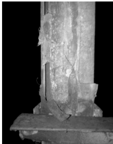
Fig. 1. Portions of the corroded filter on the measuring tube of the storage fuel tank
