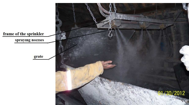
Fig. 8. First application of Bryza-1200 transfer point sprinkler (Prostański 2012c)
