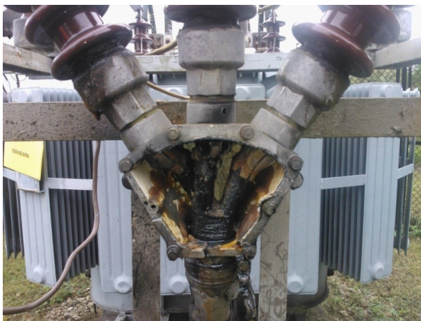
Fig. 7. View of a damaged cable head
