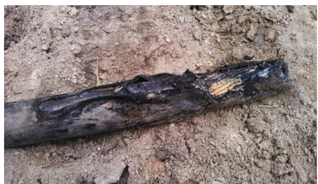
Fig. 11. A view of a damaged traction cable core
