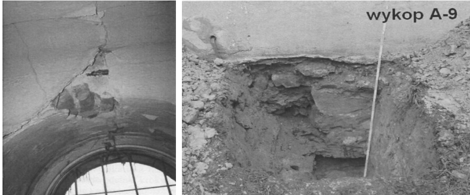
Fig. 3. Lintel with a visible crack exposing the reinforcing steel, 5 th floor (tower) [4].
