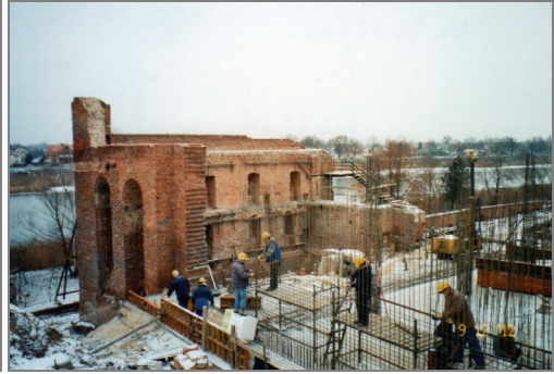
Fig. 7. The state of progress of the construction works, December 2012; the south-east side view (photograph by Z. Duda)
