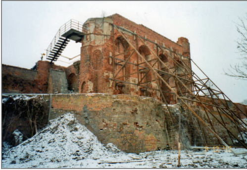
Fig. 6. The state of progress of the construction works, December 2012; the north-west side view (photograph by Z. Duda)
