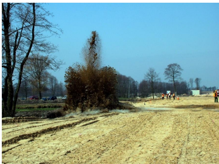
Fig. 4. The method of subsoil improving with blasting charges (A2 motorway, Kolo-Dąbnie section)
