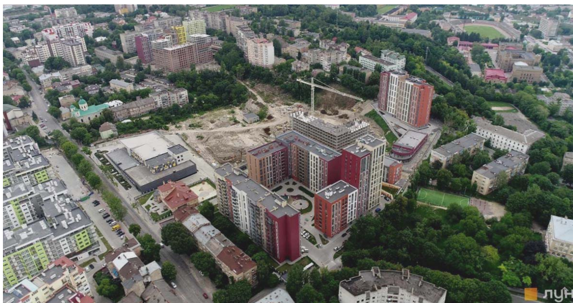
Fig. 6. Housing estate „Semycvit” at Shevchenko str. in Lviv during the construction process in year 2018.
